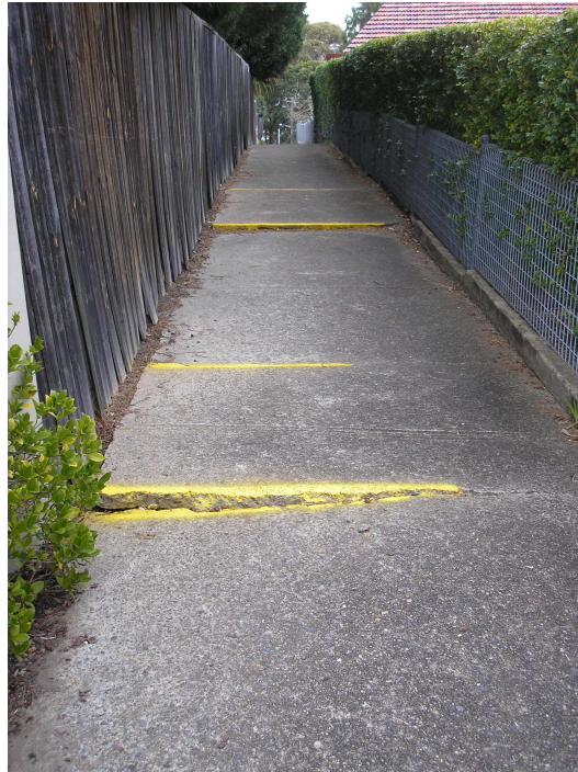
Image 41- View of drainage reserve showing condition of pavement and fencing
