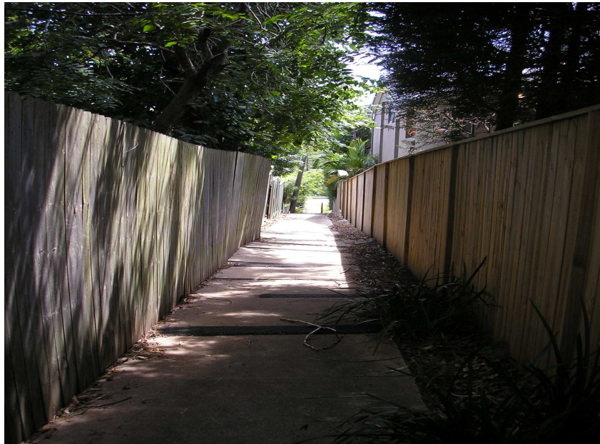
Image 44- View of drainage reserve showing condition of pavement and fencing
