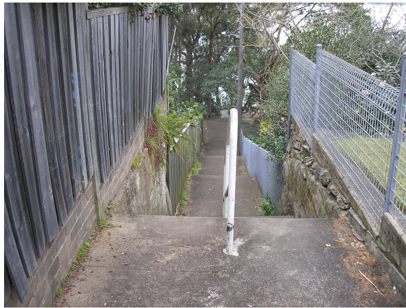
Image 42- View of drainage reserve showing condition of pavement and fencing
